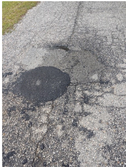
Figures 7: Patching that is failing (patches sinking and cracking) on Ponderosa Avenue
