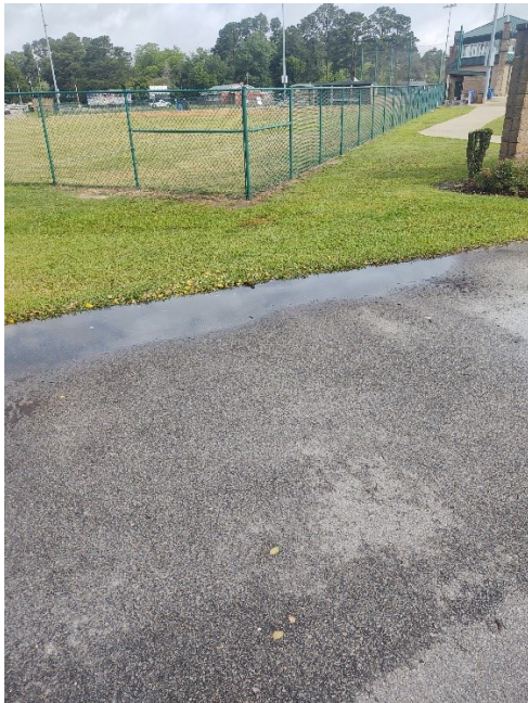
Figure 1-High shoulders holding water on parking lot
