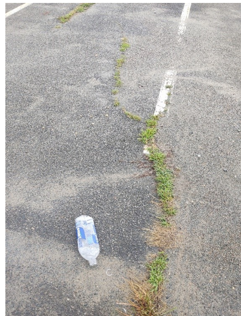
Figure 2-Grass growing in large cracks in parking lot
