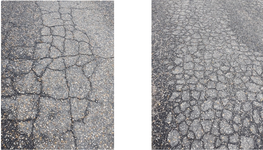
Figures 3 & 4: Fatigue Cracking as seen on W. Harnett Street and S. King Avenue
